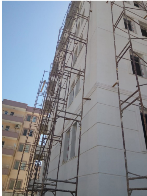
Figure 2. Final surfacing of the facade, made of acrylic based with silicon admixture
